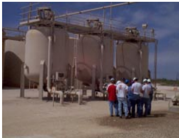
Filters at Chevron's Eunice Monument South Unit
