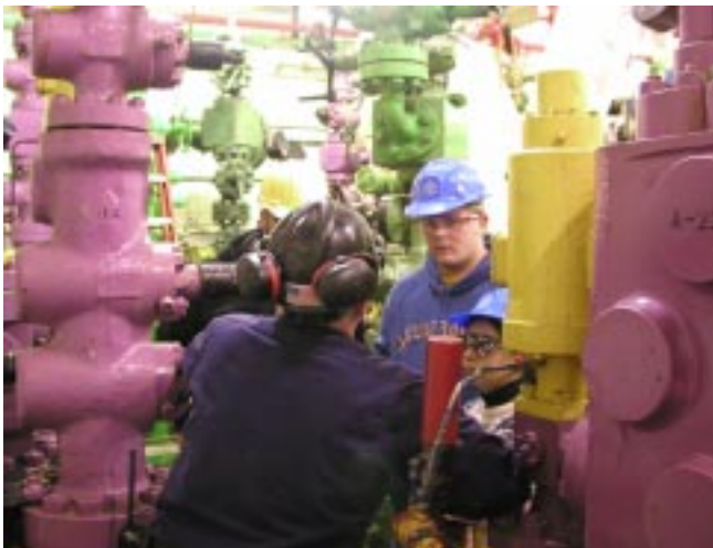
Inside the wellhead room
